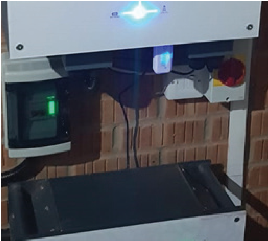
Example of GivEnergi system
